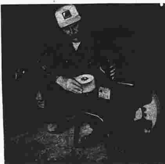
This generator owner knows when to follow his maintenance checklist - before he needs emergency electrical power on a stormy winter night. He is removing the air filter cover in order to clean the filter.
